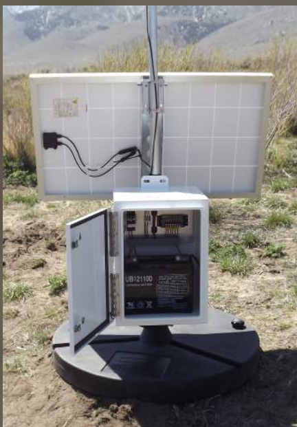
Trickle Charge Battery System With Portable Mast
